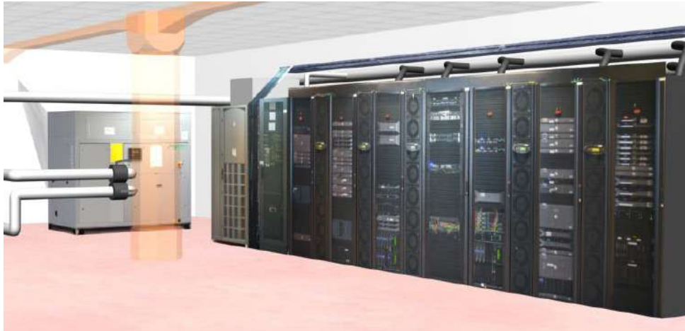
Figure 3. Le datacenter belfortain.
